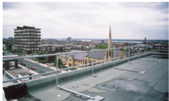
Figure 40 Permanent guard rail retrofitted during refurbishment work. Similar protection can be included in initial designs (image courtesy of Safesite Limited)
