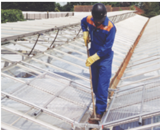
Figure 12 Valley walker used during gutter cleaning. This provides a protective mesh covering to either side of the operative, which moves progressively along the roof as the worker moves forward. The protective covering eliminates the risk of a fall through the fragile material (image courtesy of Safesite Limited)
