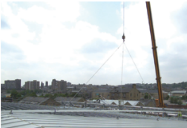
Figure 36 (a)–(c) 24-m long roof panels being mechanically lifted from ground level and installed on roof
