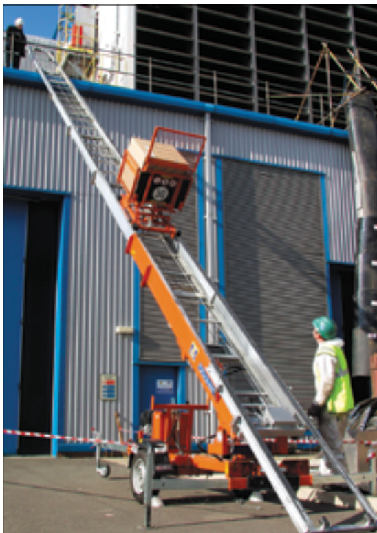
Figure 4(a) Industrial hoist (images courtesy of HSS)
