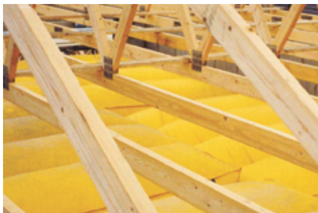
Figure 14(b) Airbags being used as a fall mitigation measure during roof work (image courtesy of Airtek Safety Products Ltd)
