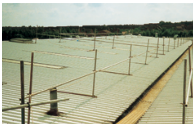
Figure 20 Demarcation barriers on a large, non-fragile roof preventing access to the adjacent roof lights. The roof lights are at least 2 m from the barrier
