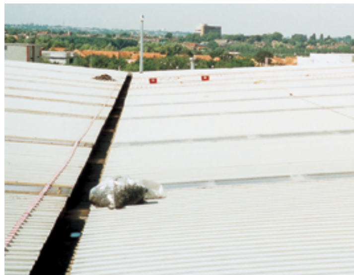
Figure 27 In some light conditions, it is difficult to distinguish the roof lights from the metal sheets on this type of roof. The valley gutter is very narrow and the roof lights extend down to gutter level. Both of these features increase the risk during cleaning, maintenance and refurbishment
