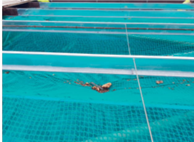
Figure 7 Debris netting used in addition to safety netting may enable work to be carried out safely below roof workers (Image courtesy of Highersafe (North East) Ltd)
